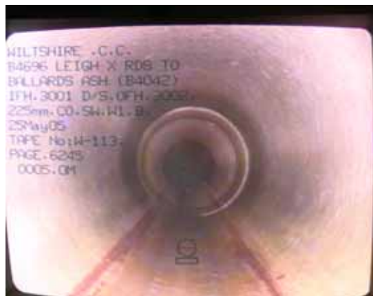
Example of how the video evidence can also show that the drainage system is in good condition
